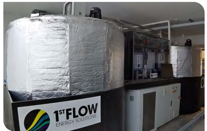
Vanadium redox-flow battery with insulation. (KIT/Felix Schofer)
